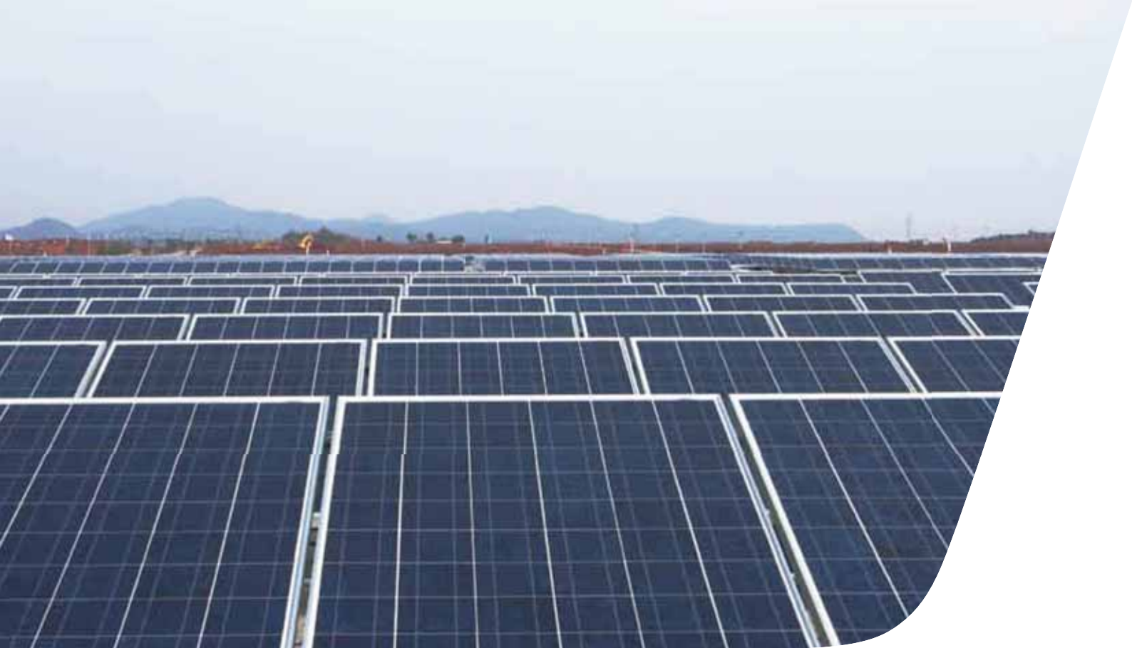
Photo Courtesy: LDK Solar Power Tech./ Location: Xin Yu, China/ System Size: 2MW/ LDK factory rooftop application
